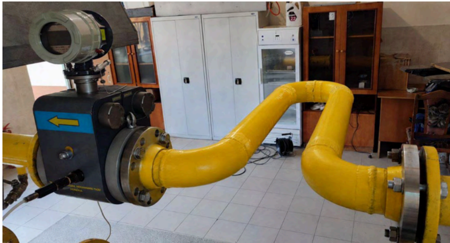
Combined local resistance DN80 installed in the horizontal plane
