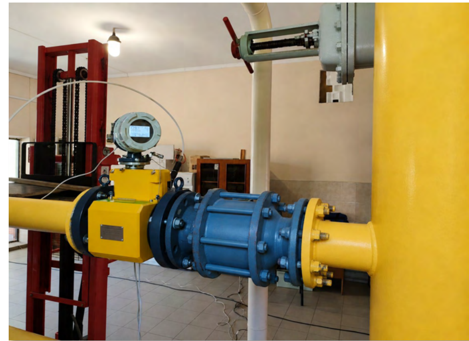
GFA424 DN100 installed directly downstream of a valve and a tee with a change in flow direction and a sharp constriction
