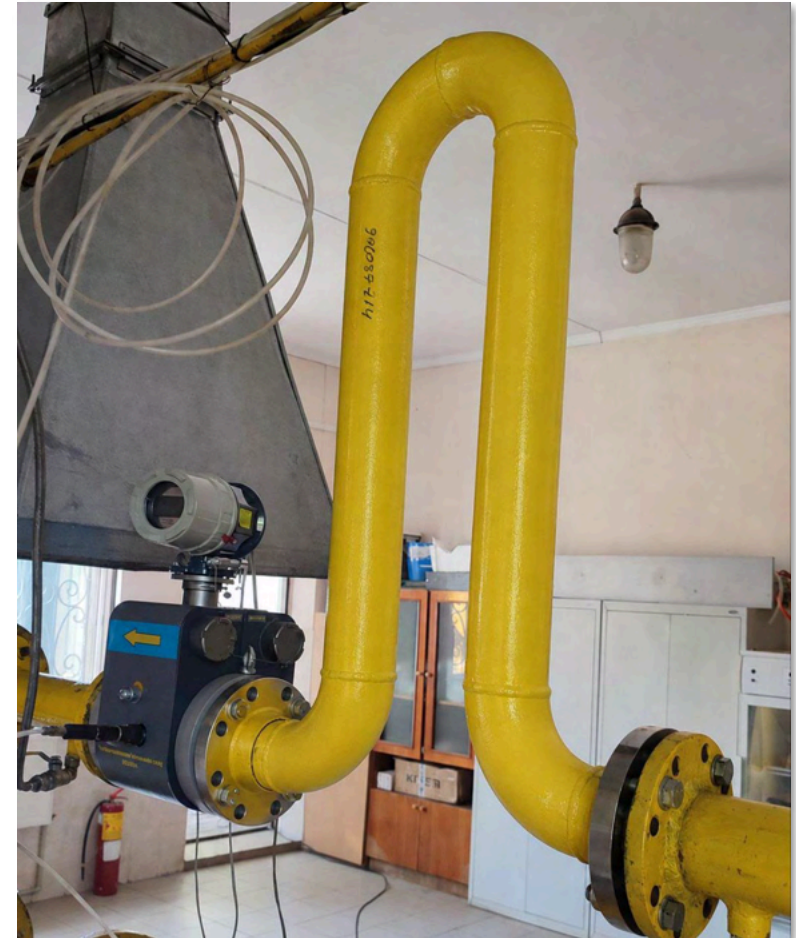
Combined local resistance DN80 installed in the vertical plane
